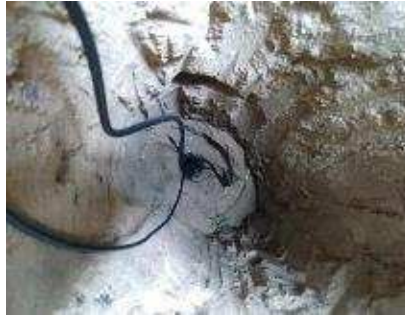
Figure 99. Conduit hole within the hole
