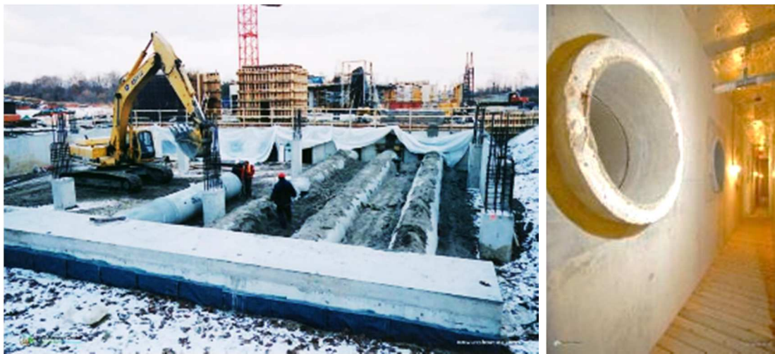
Figure 56. Earth Rangers Centre, Earth Tubes 68
