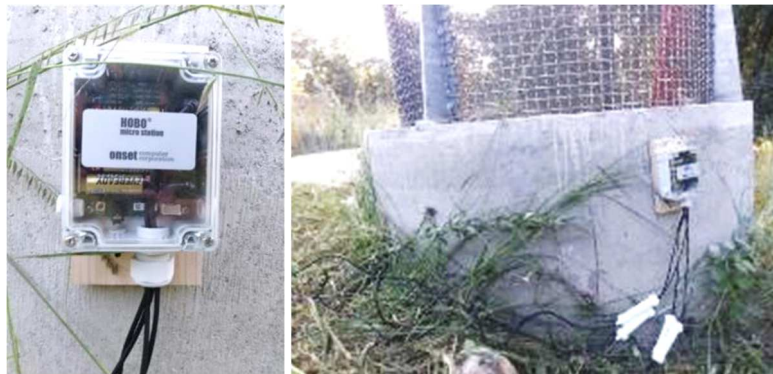
Figure 95. Micro station attached to the manhole wall
